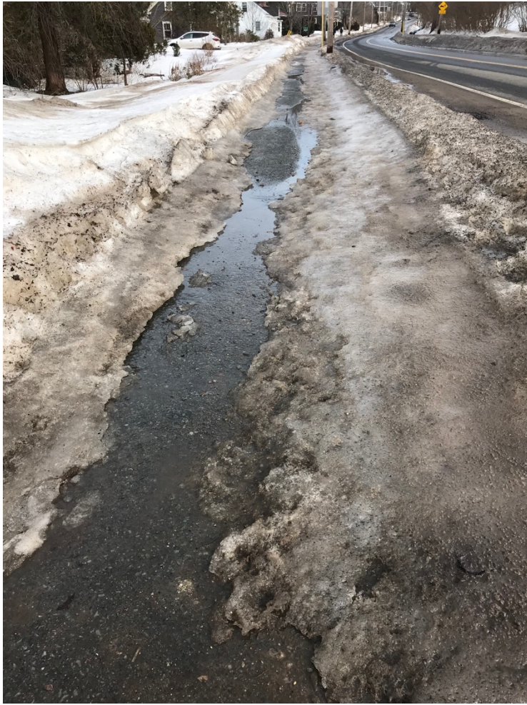
IMG8977 -Feb 17, 2.31pm – Snowbanks blocking drainage to curb. Attention still needed although in general better clearance and use of sand done after storm Feb 14.
