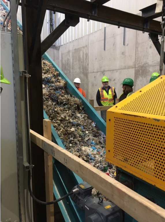
Shredded garbage on a conveyor belt.
