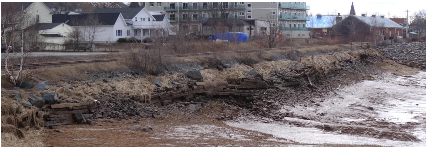
Figure 8.3: Erosion on the Bank by the Railroad
