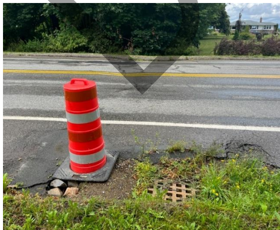
Road Surface Degradation
