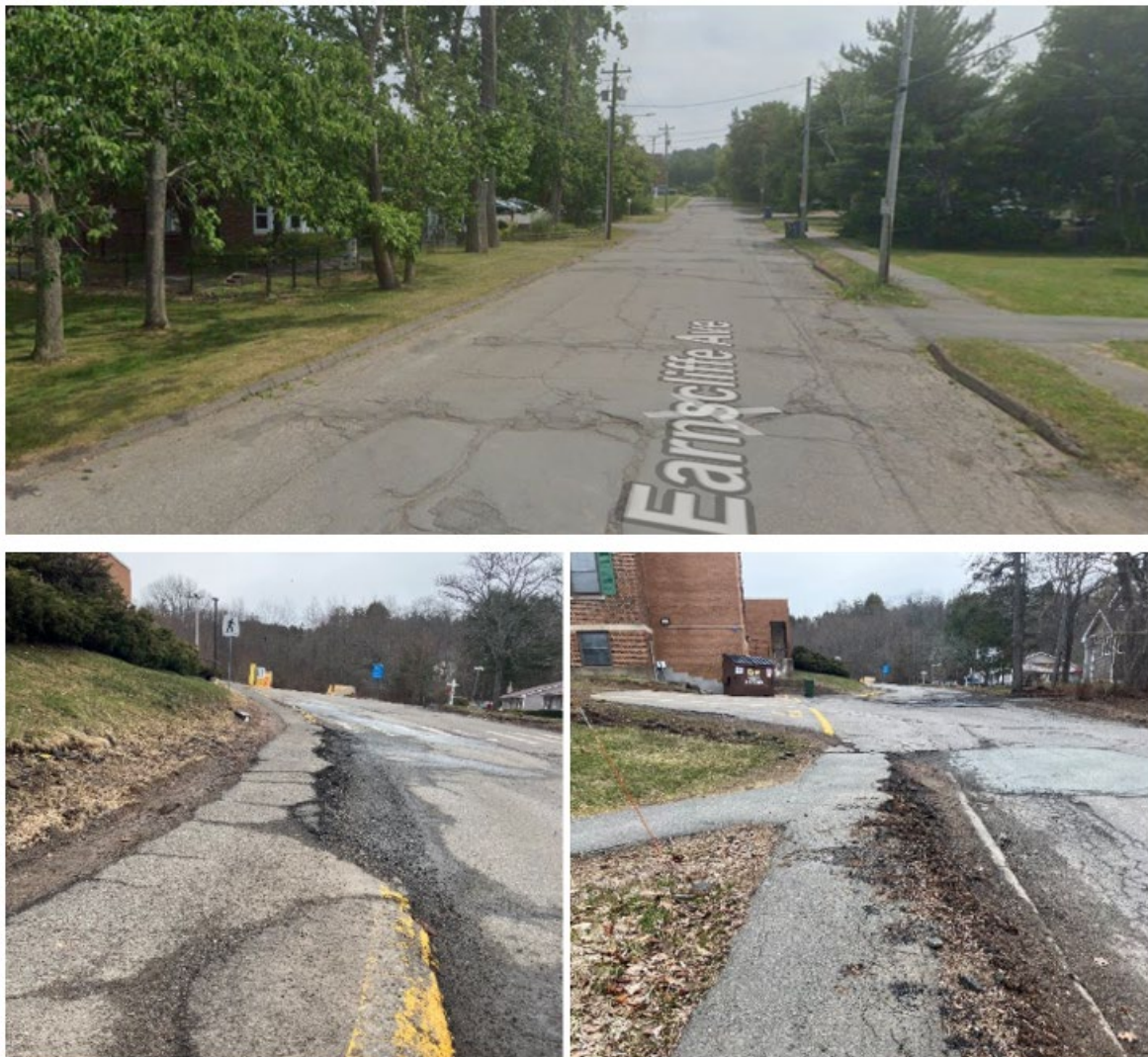
Figure 1 – Street and Sidewalk condition examples
