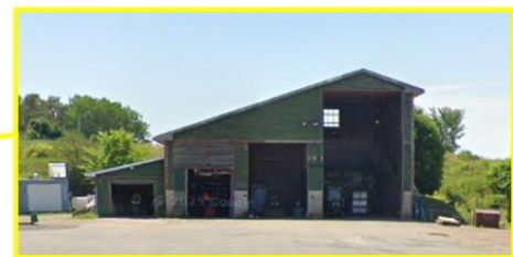
Proposing 2026 to refurbish the existing salt shed at public works for storage and work area
