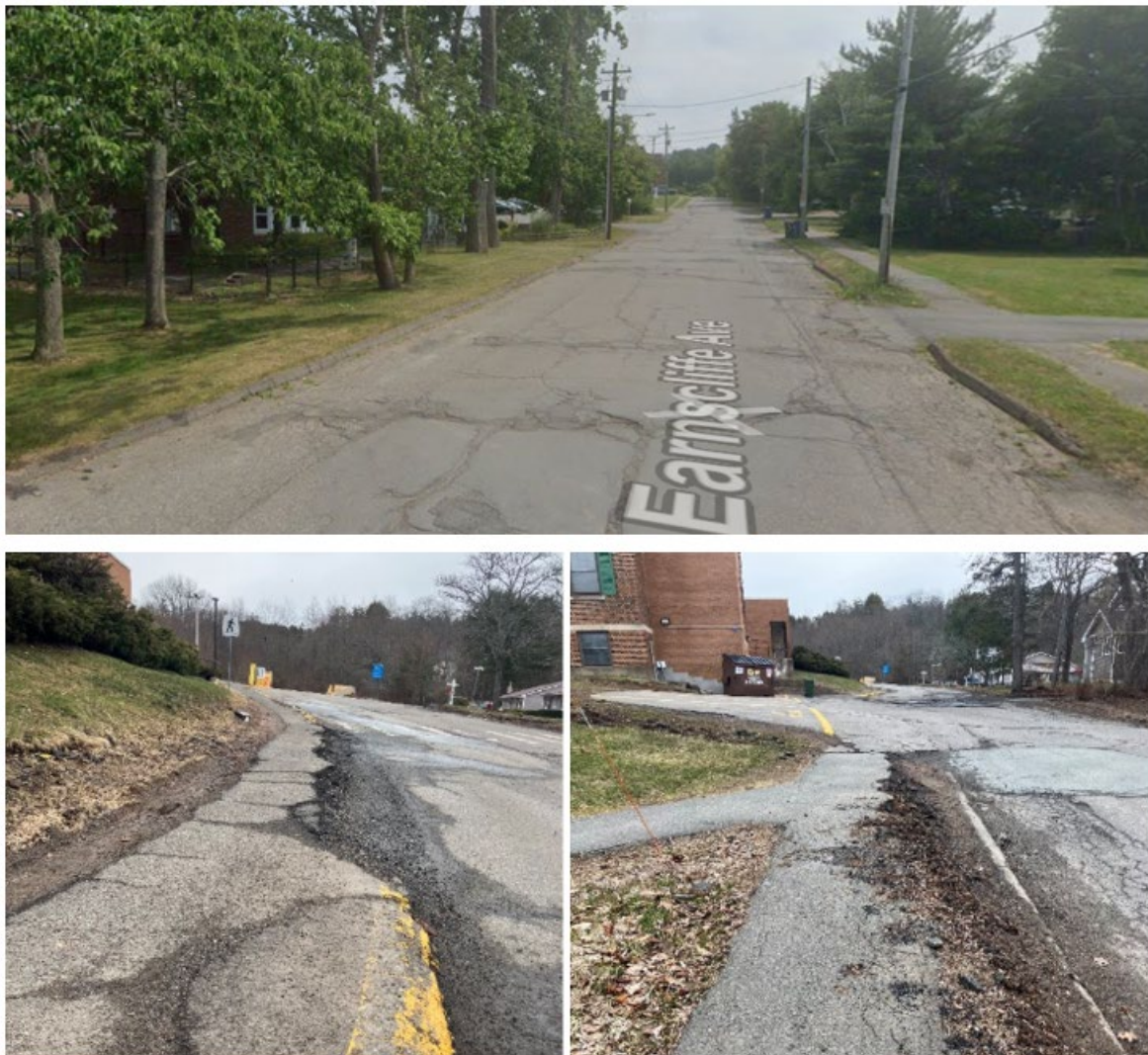
Figure 1 – Street and Sidewalk condition examples
